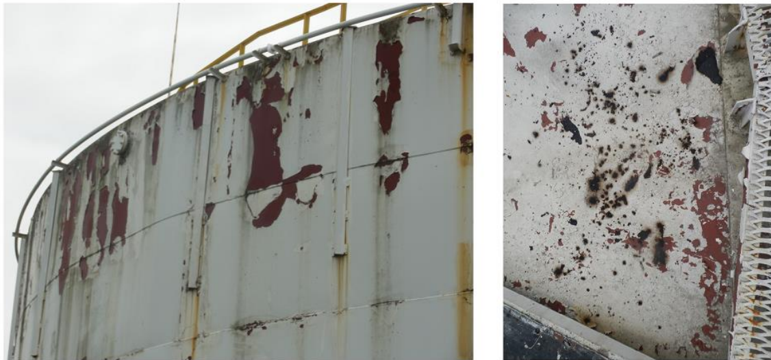
Fig.. 2. Corrosion of tank structures.
