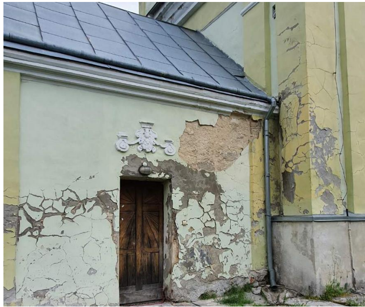
Figure 8. Damage to the facade and blind area.
