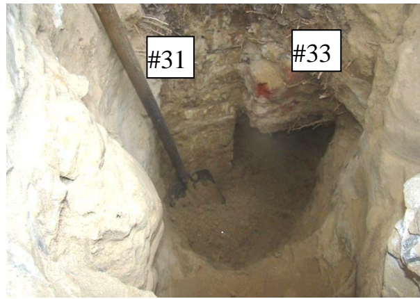
Figure 3. The sole of the foundation of building #31 is located 0,5 m below the sole of the foundation of building #33
