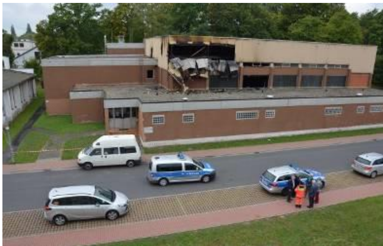
Fig.4. Burned building for migrants. Wertheim [19]
