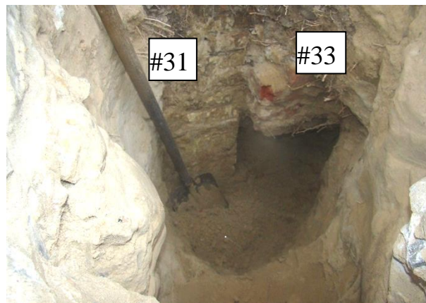
Figure 3. The sole of the foundation of building #31 is located 0,5 m below the sole of the foundation of building #33
