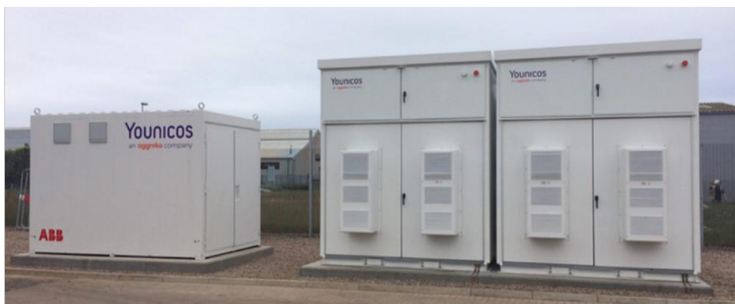
Figure 19. High capacity batteries
