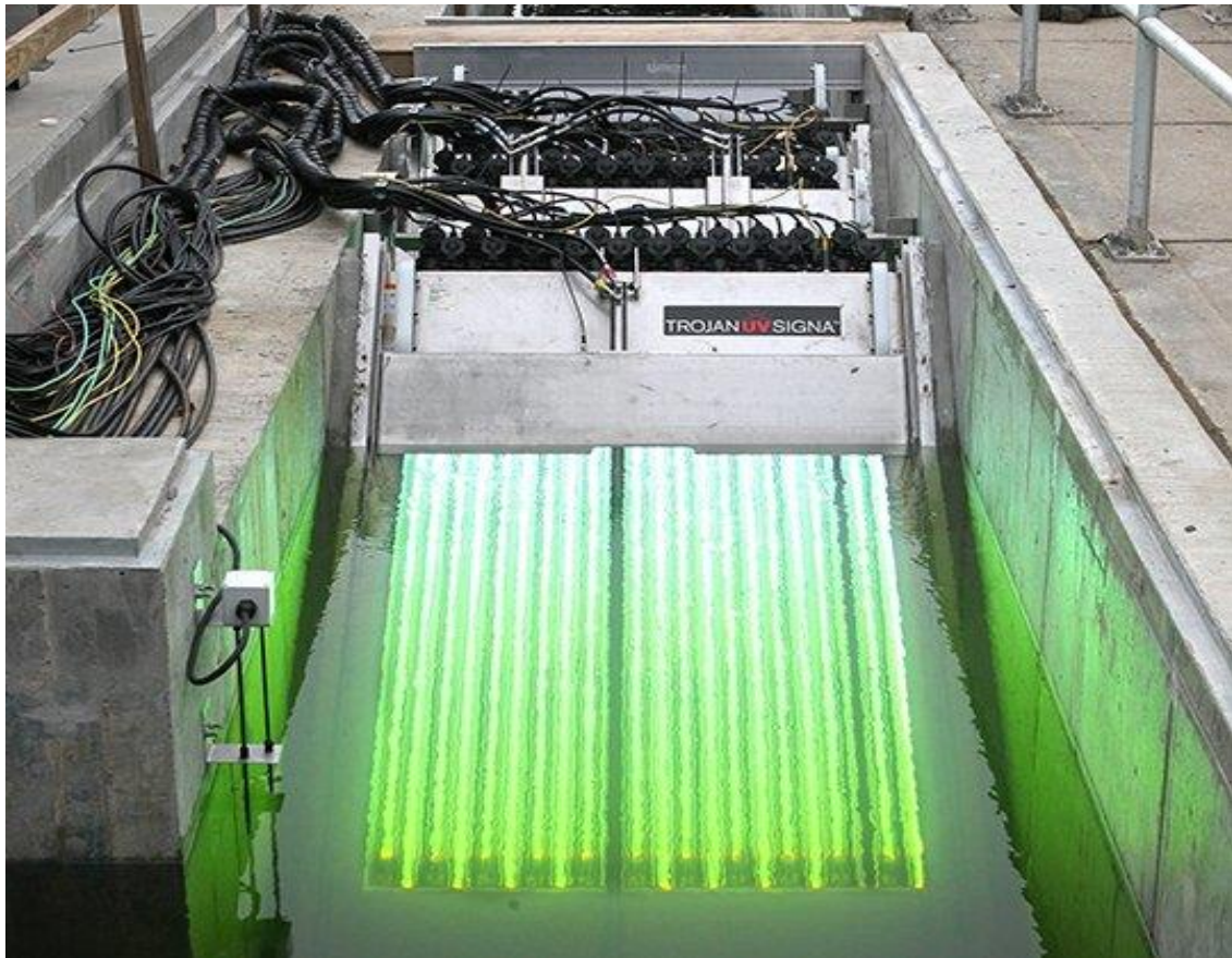
Figure 5. The example using of mercury lamps in UV disinfection
