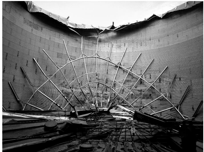
Figure 7. Hanging of the destroyed elements of the load-bearing structures of the conical coverings of silo #5 on the contour of its wall
