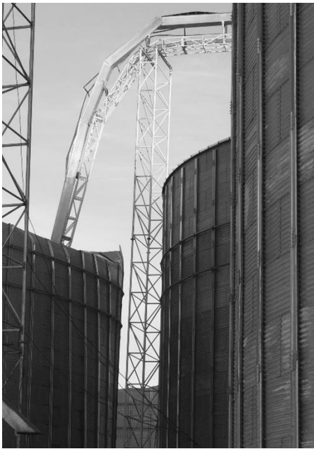
Figure 6. Lattice vertical rack between silos #4 and #6 and continuous lattice truss of the conveyor gallery
