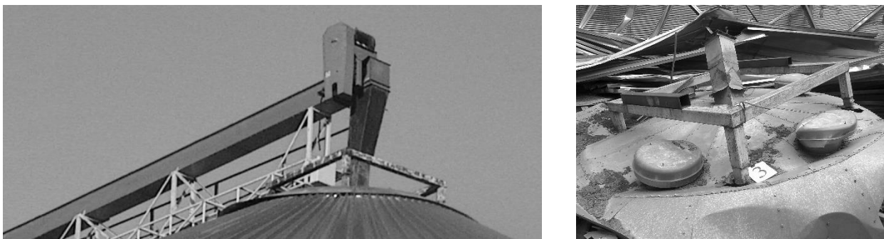
Figure 5. Rigid fastening of the lattice trusses of the conveyor galleries above the silos through the "chair" to the central ring of the conical cover
