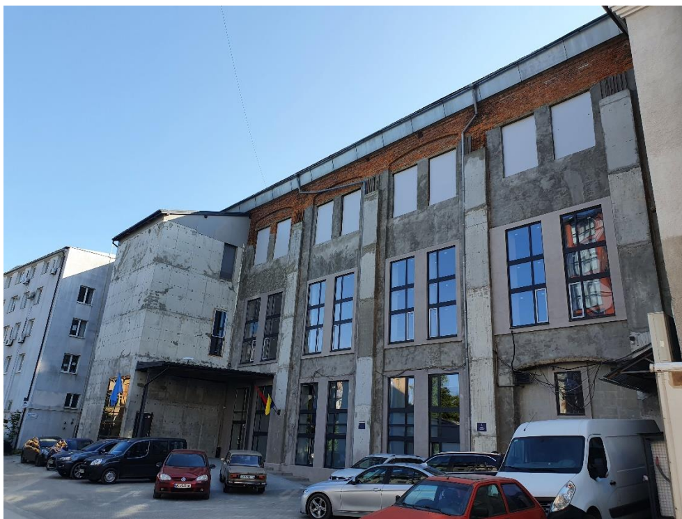
Figure 12. General appearance of the facade after reinforcement (at the stage without adding floors)
